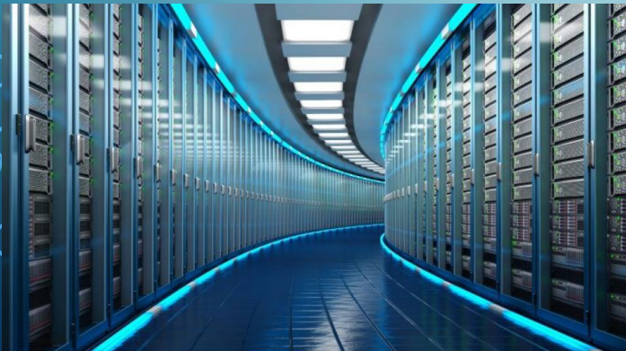
It is predicted that 175 zettabytes of data will be produced by 2025, which will make data centers to continue to play a vital role in the ingestion, computation, storage, and management of information.
